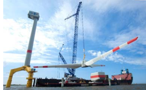
A crawler crane lifting the blades for assembly of an offshore wind turbine.
