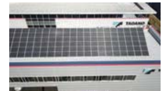
Solar panels installed at Advanced Technology Research Center
