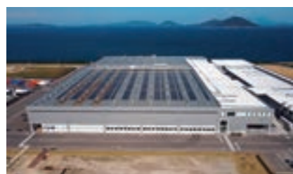
Solar panels installed at Kozai Plant
