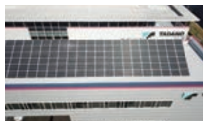
Solar panels installed at Advanced Technology Research Center
